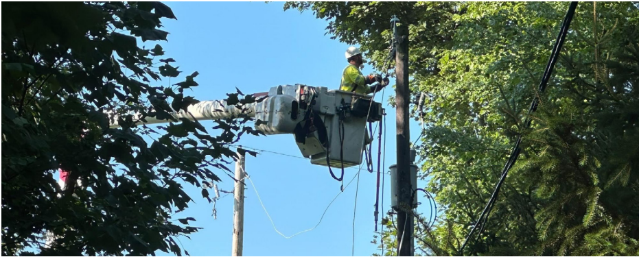
Our lineworkers worked around the clock during Tropical Storm Debby. We brought in an additional 1000 workers from our first-tier contractor list. With significant damage across our 29-county service territory, our team restored power to over 71,000 customers at hundreds of outage locations.
